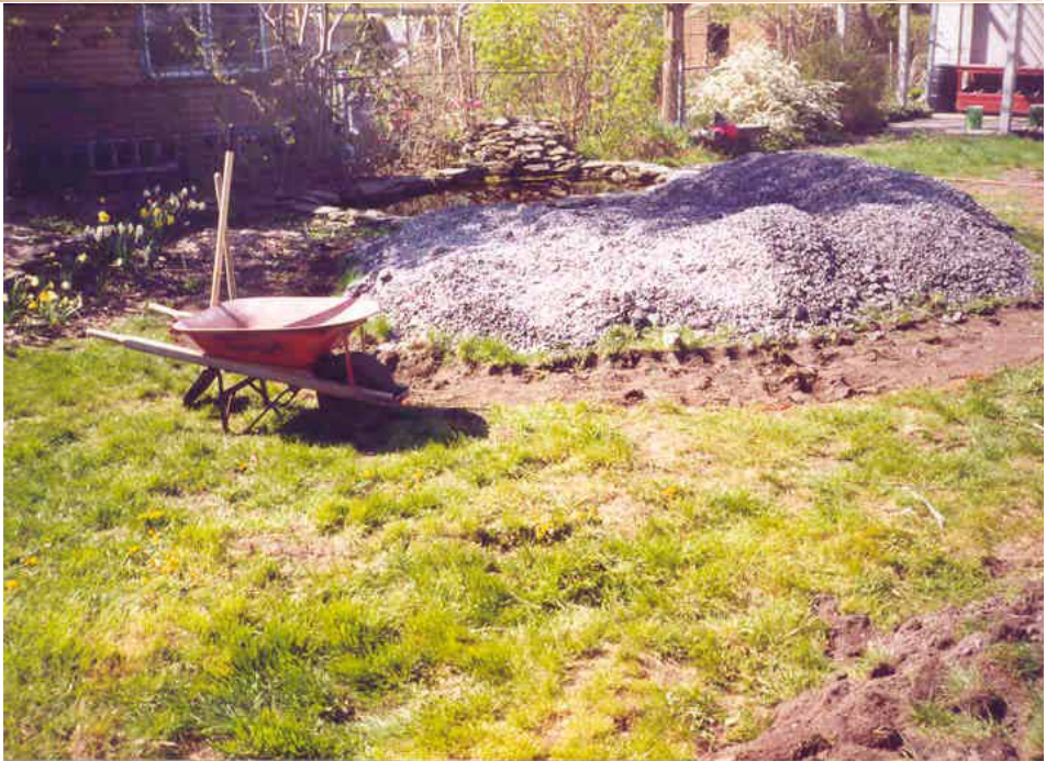
Top: The designs for the garden showing the different types of gardens included, and the different materials used for the construction. Bottom: Designs on paper become reality as construction begins.
